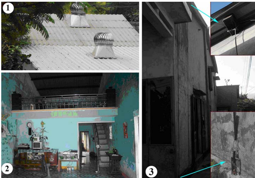
Figure 26. The reinforce methods in Sections 29&30 (1). Tie up the roof; (2) The “family shelter”; (3) Fixing the purlins
